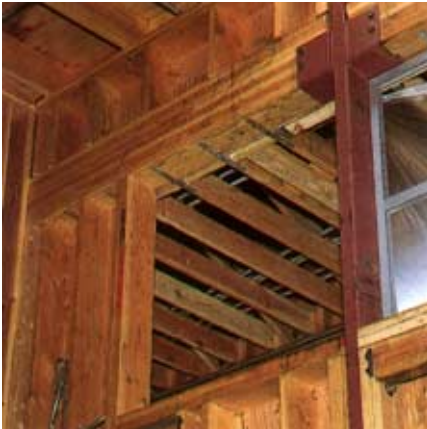
Glulam header provides strength above a window.
