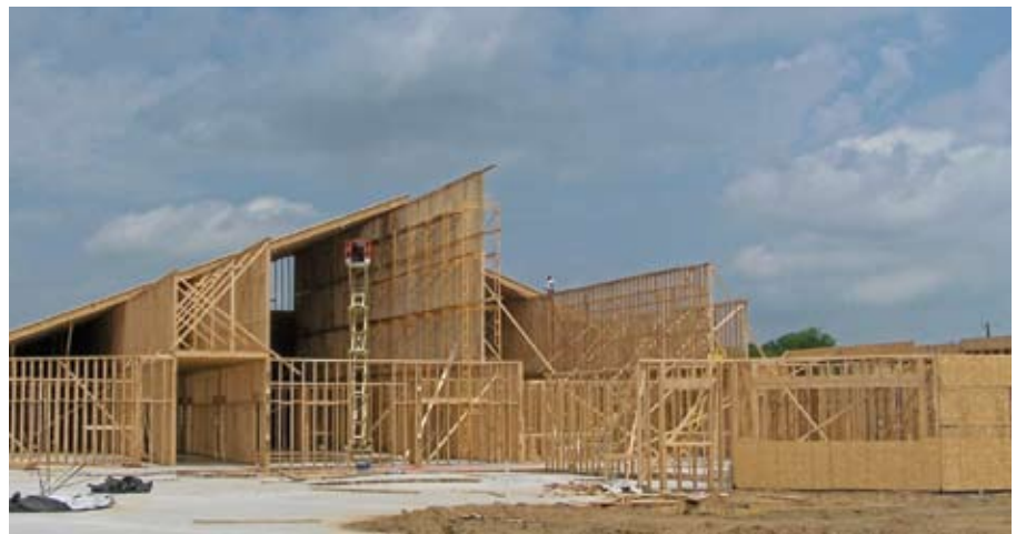
Constructed of all wood, Gunter Primary School used a variety of APA trademarked engineered wood products.
