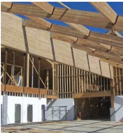
Supporting the roof framing, this large glulam beam in the school's cafeteria is APA trademarked from Standard Structures, Inc. The glulam, measuring 12 inches wide by 7 feet deep and 82 feet long, also supports a vertical wall directly above.
