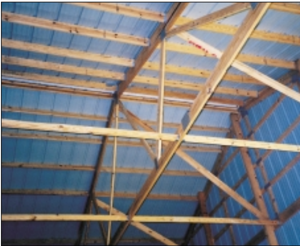
Purlins placed flush with the top of trusses simplify installation of roof sheathing.
