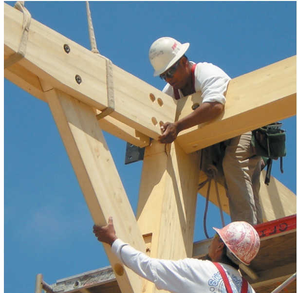
All holes, notches, and tapered cuts must be approved by the engineer or architect.
